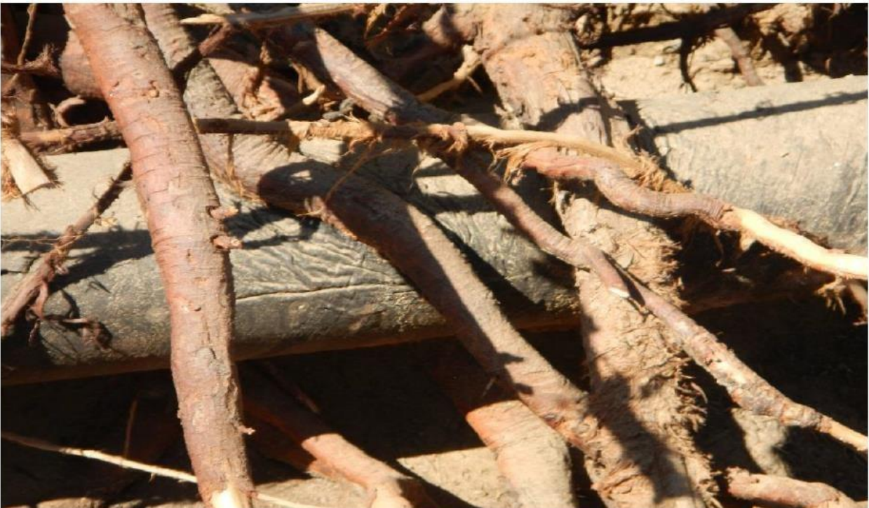
Figure 2. Tree roots causing coating damage to RWVIM-107-13 (Weber Lane) pipeline. (Figure 3 from Dynamic Risk 2015).
